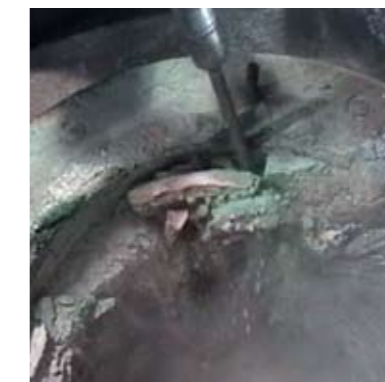
The upper ring of the crucible is to remove with an air hammer.
